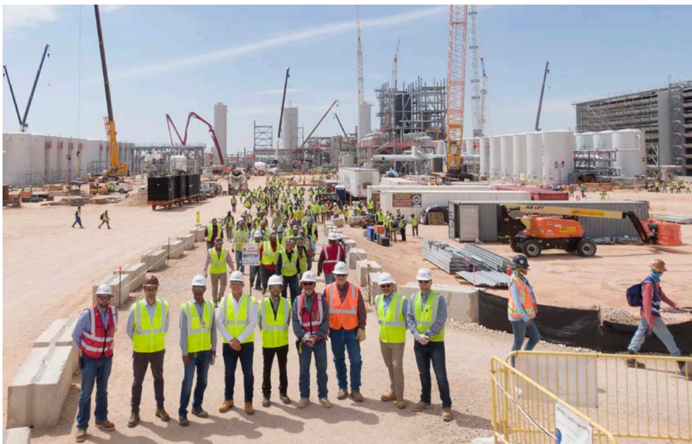
Worley is currently providing EPC services for 1PointFive's STRATOS facility, which will be the largest Direct Air Capture (DAC) facility in the world
