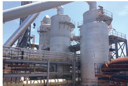
Brick Lined Acid Towers
