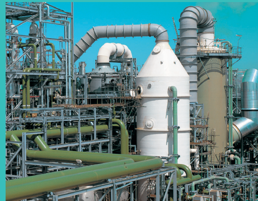
Sulphuric Acid Regeneration Plant
